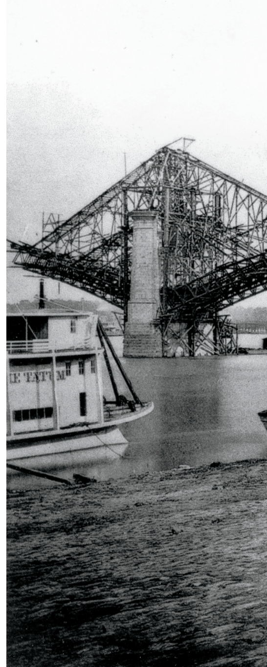
Supported by temporary towers and cables, the steel tubes cantilever outward from the abutment and the west river pier. Robert Benecke, Woodward, History , plate XLIII
